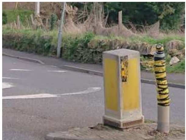
Damaged street furniture at Academy Drive
