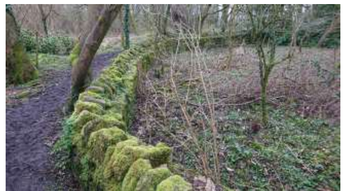
Wall to the north-west of the Nature Area—restoration should be considered for the sections which have fallen into disrepair
