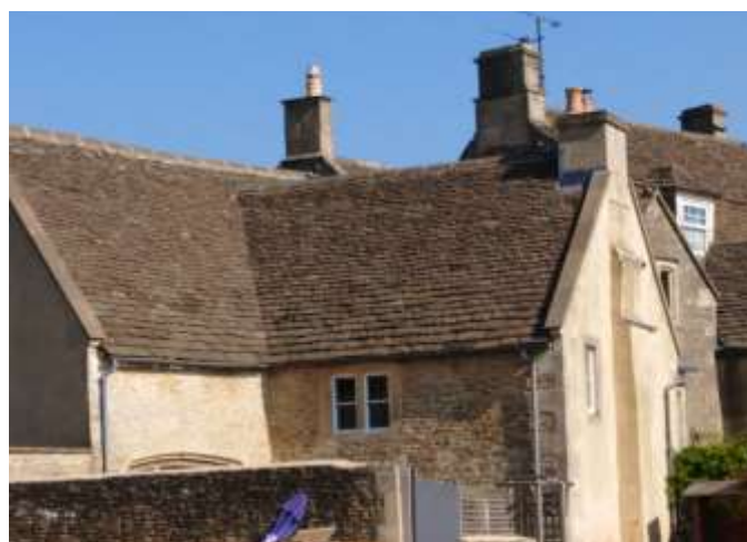
Another rebuilt stump without shaft (on gable at right)
