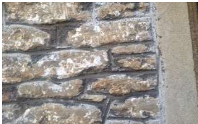
Recessed pointing at Pickwick Manor 1920
