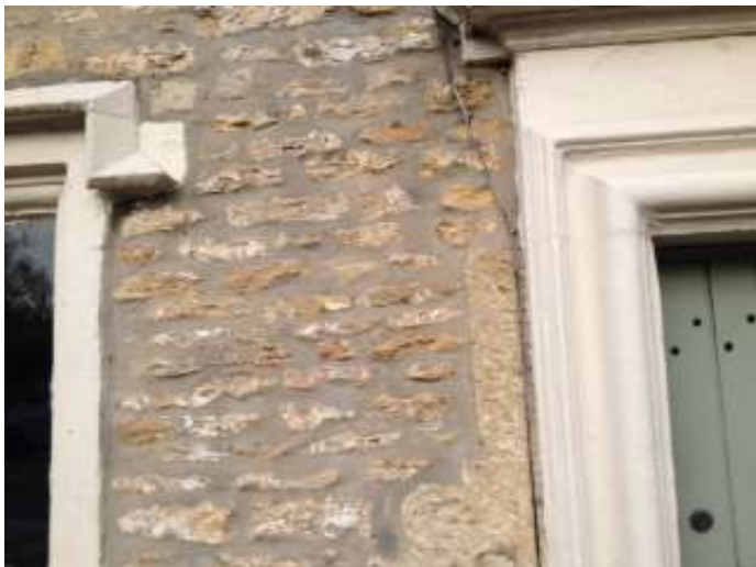
Cement rich pointing c 1978. The south end of the Hare and Hounds was previously roughcast.
